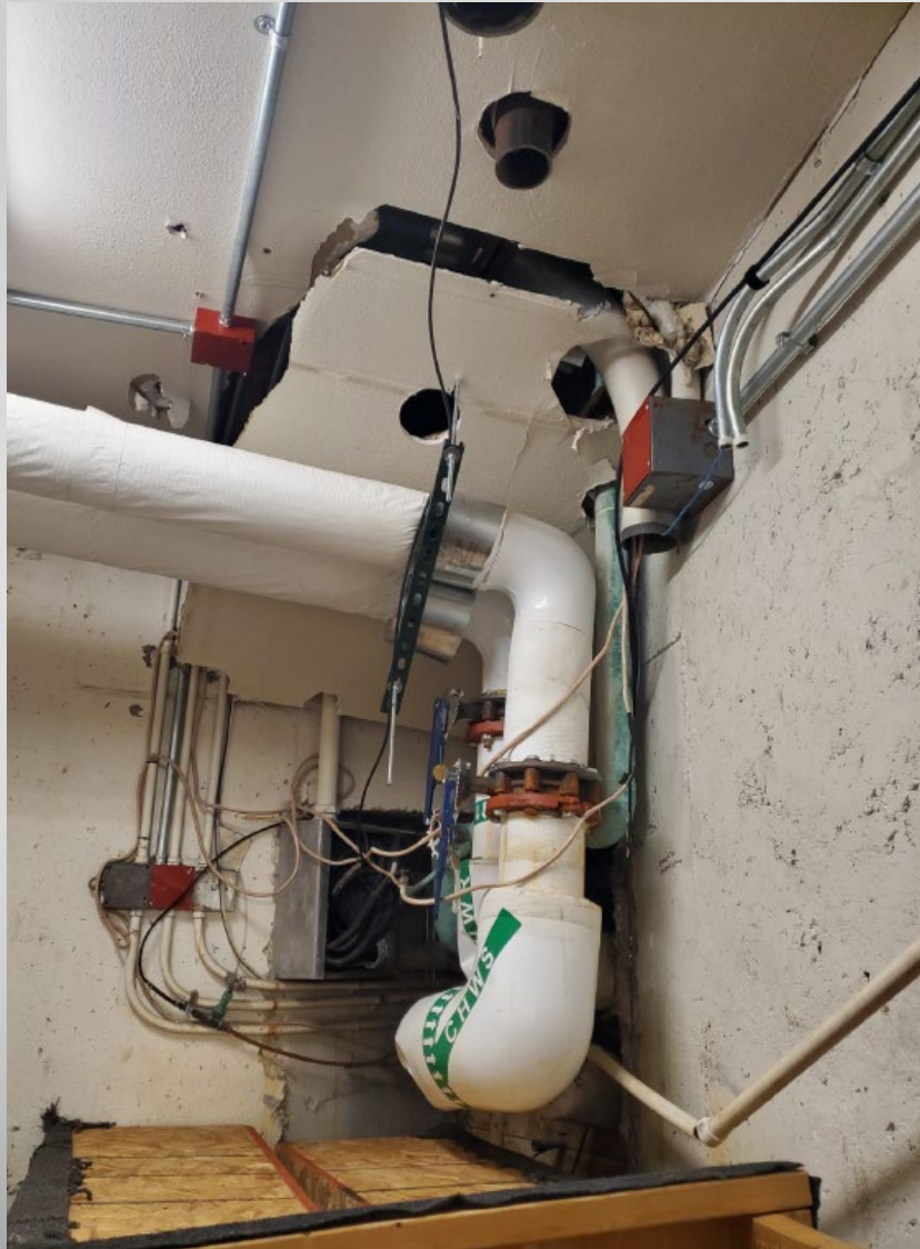
HEFLEY – Supply Lines (Damaged Ceiling)
