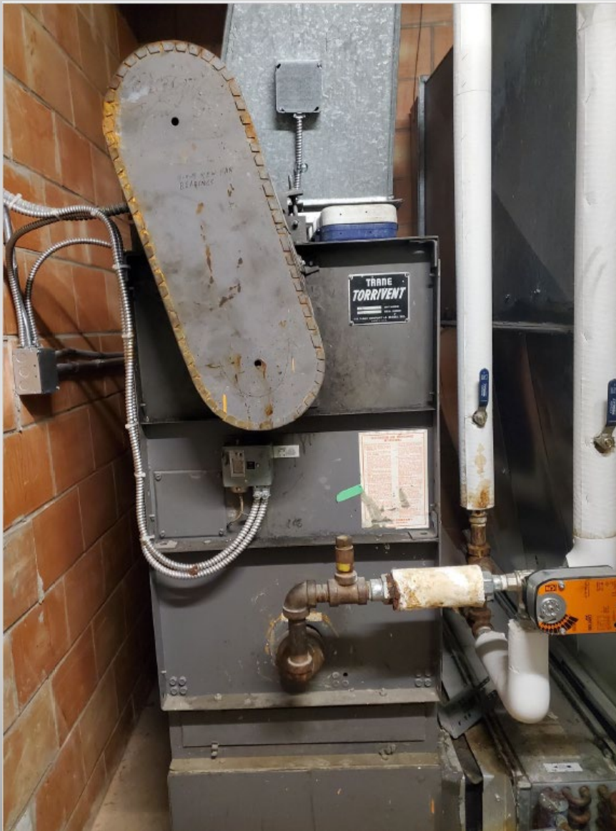
HEFLEY – Air Handling Unit
