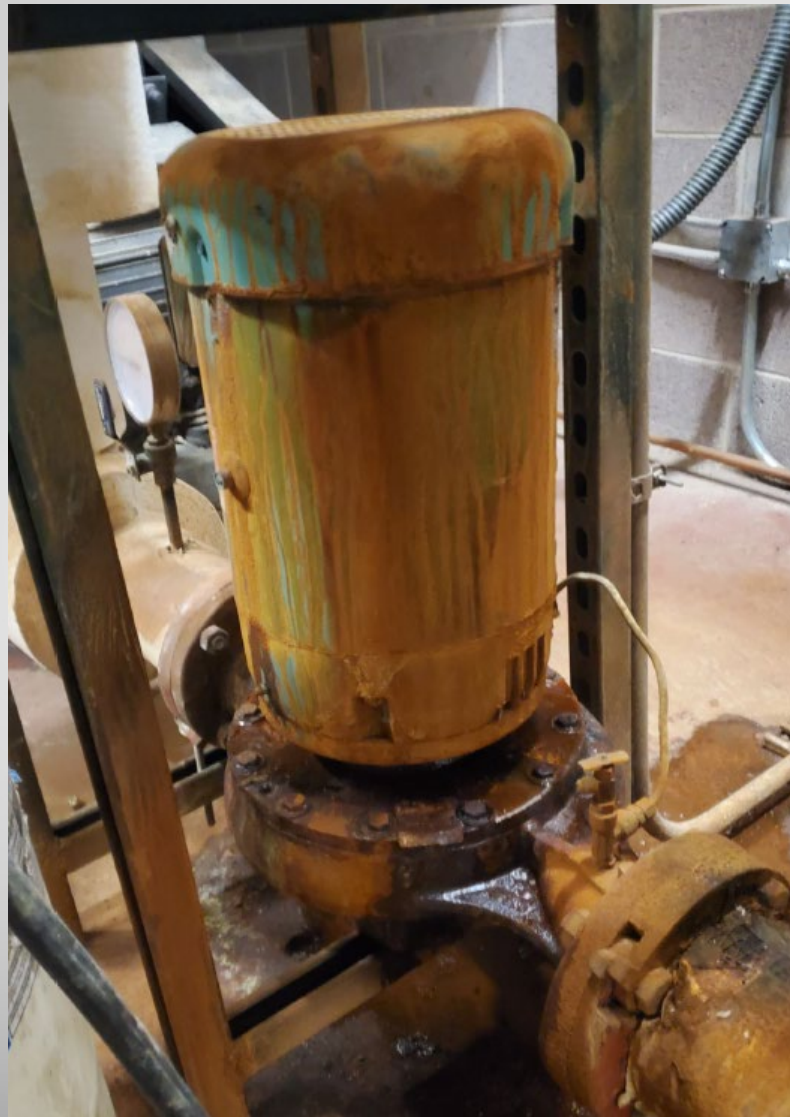
HEFLEY – Main Supply for Hydronic Heating System
