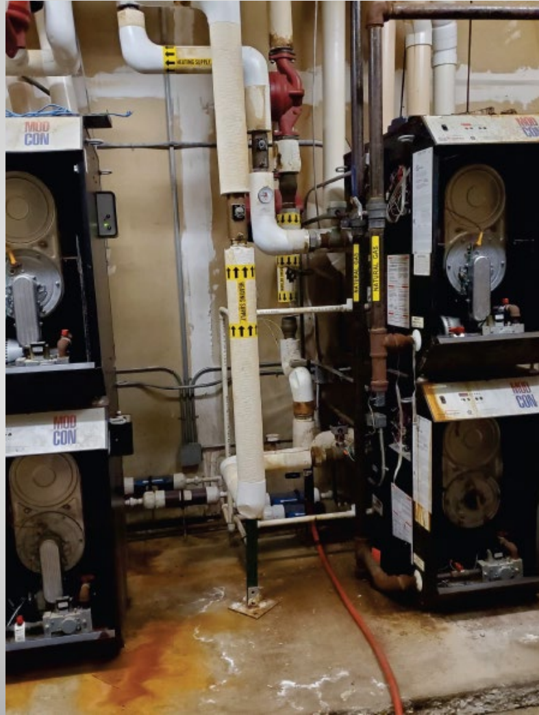
WEISS – Failed Boilers
