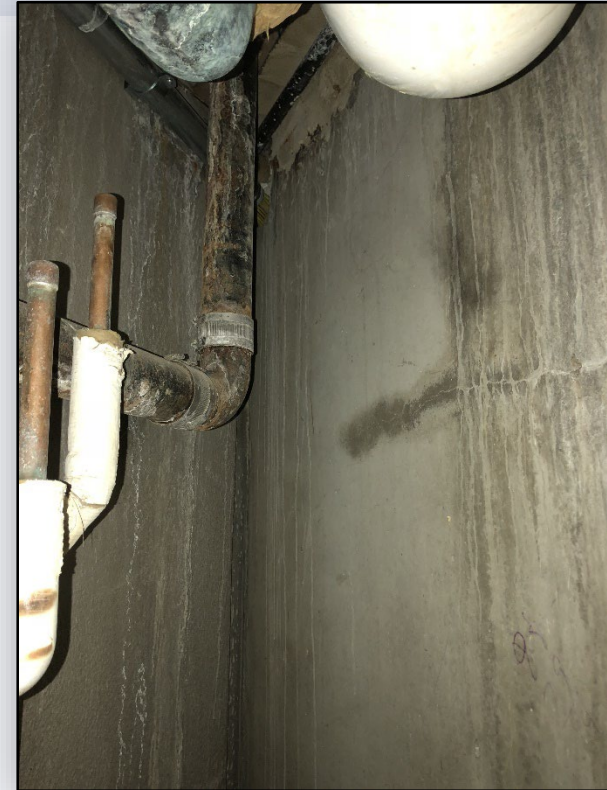
Arkansas Valley Correctional Facility Corroded electrical & plumbing systems resulting from shower drain leaks
