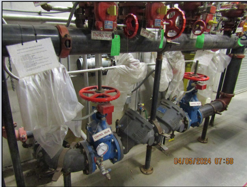
Denver Reception & Diagnostic Center Fire protection system valves
