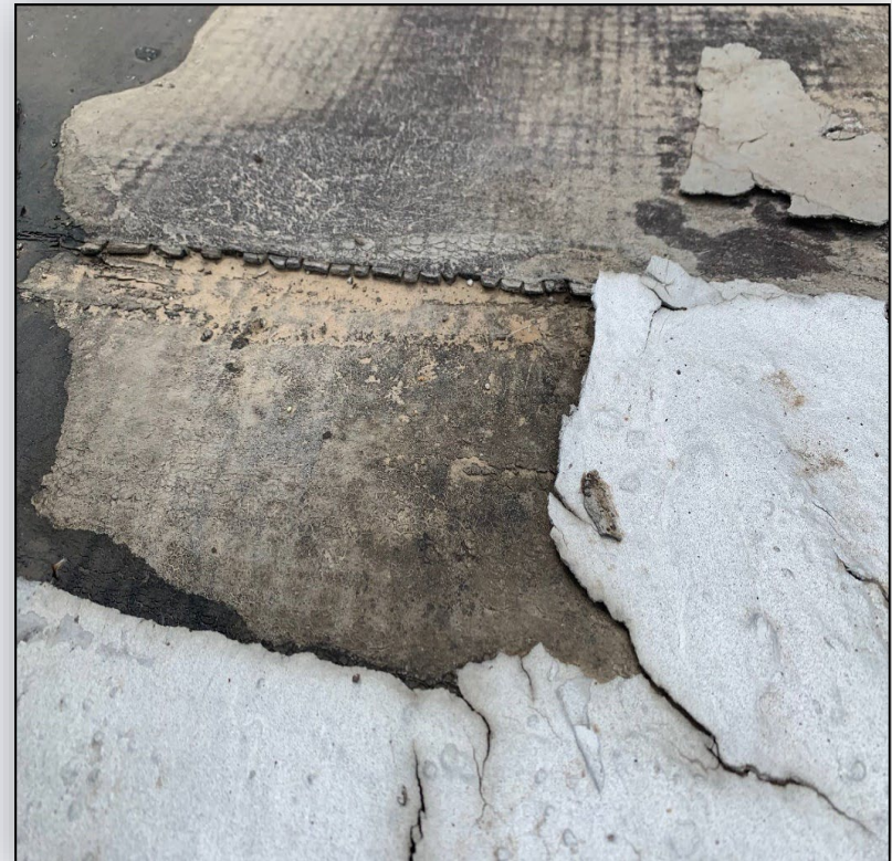
Buena Vista Correctional Facility Failed roof conditions
