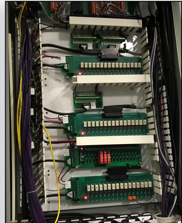
Colorado State Penitentiary Antiquated control panel
