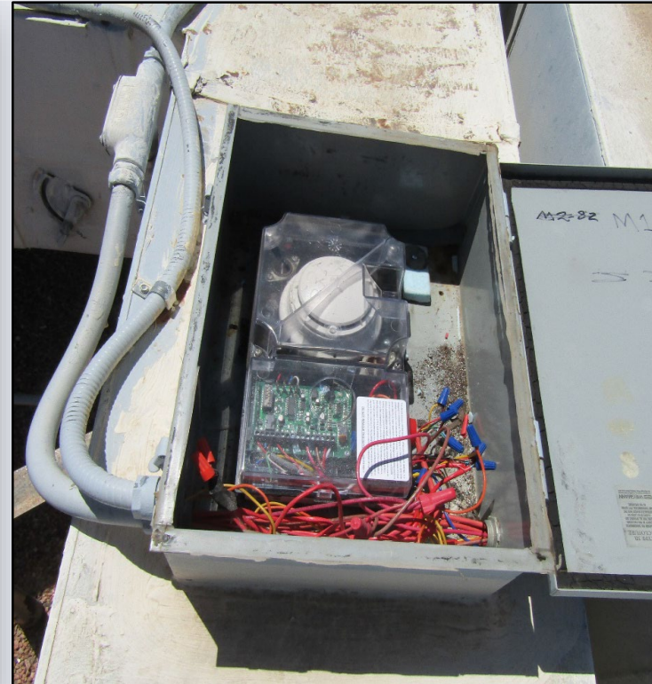
Fremont Correctional Facility Fire alarm distribution conditions
