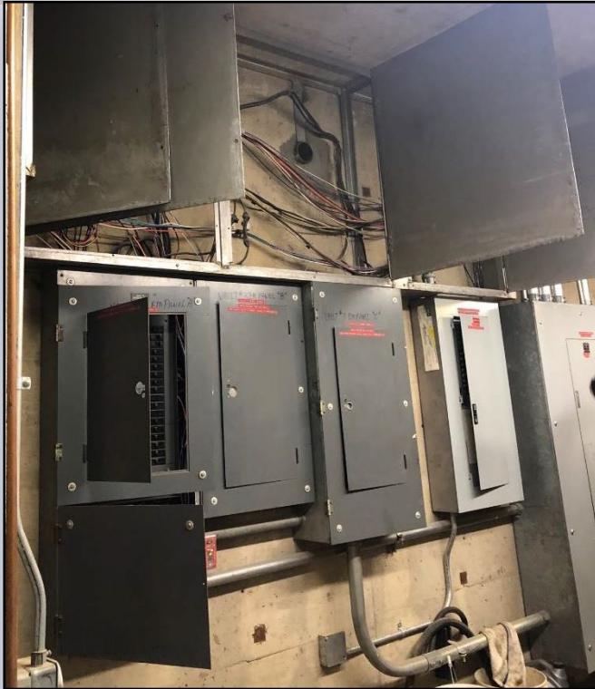
Fremont Correctional Facility Electrical Panel Distribution
