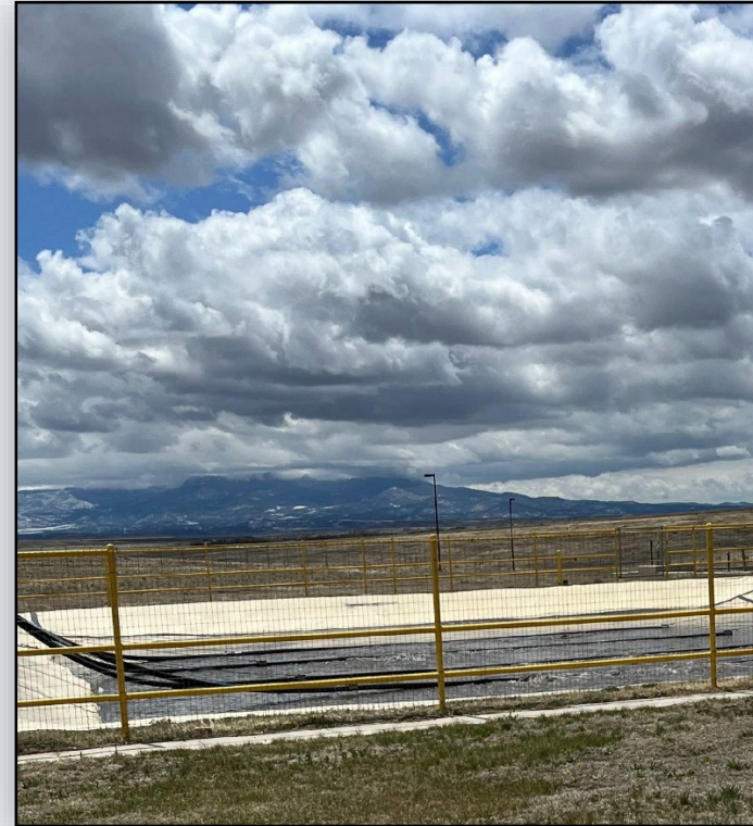
Trinidad Correctional Facility WWTF treatment pond condition
