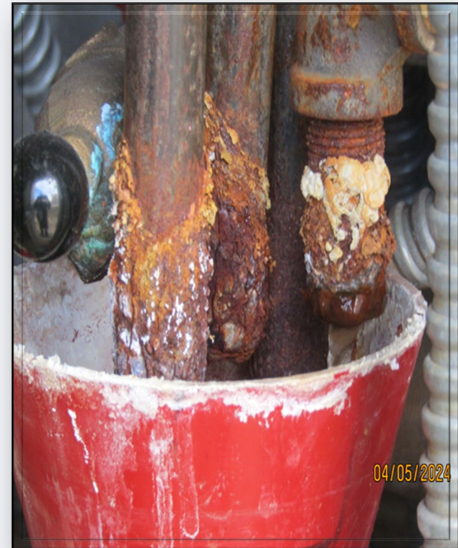
Denver Reception & Diagnostic Center Corroded fire suppression
