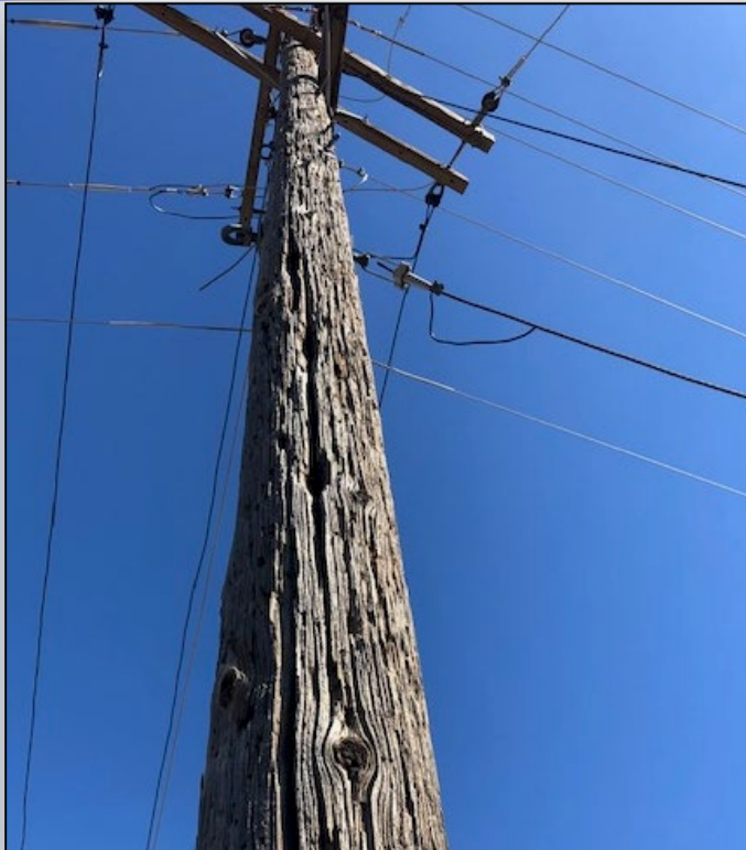
East Canon City Prison Complex Electrical distribution conditions
