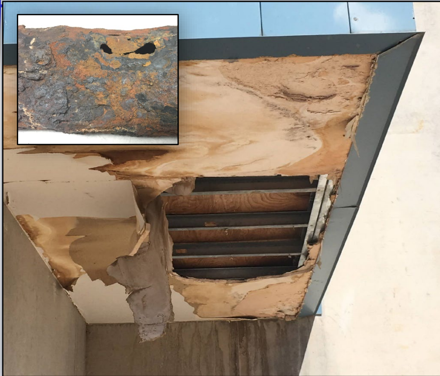
Sterling Correctional Facility Steam condensate leaks damaged exterior soffit
