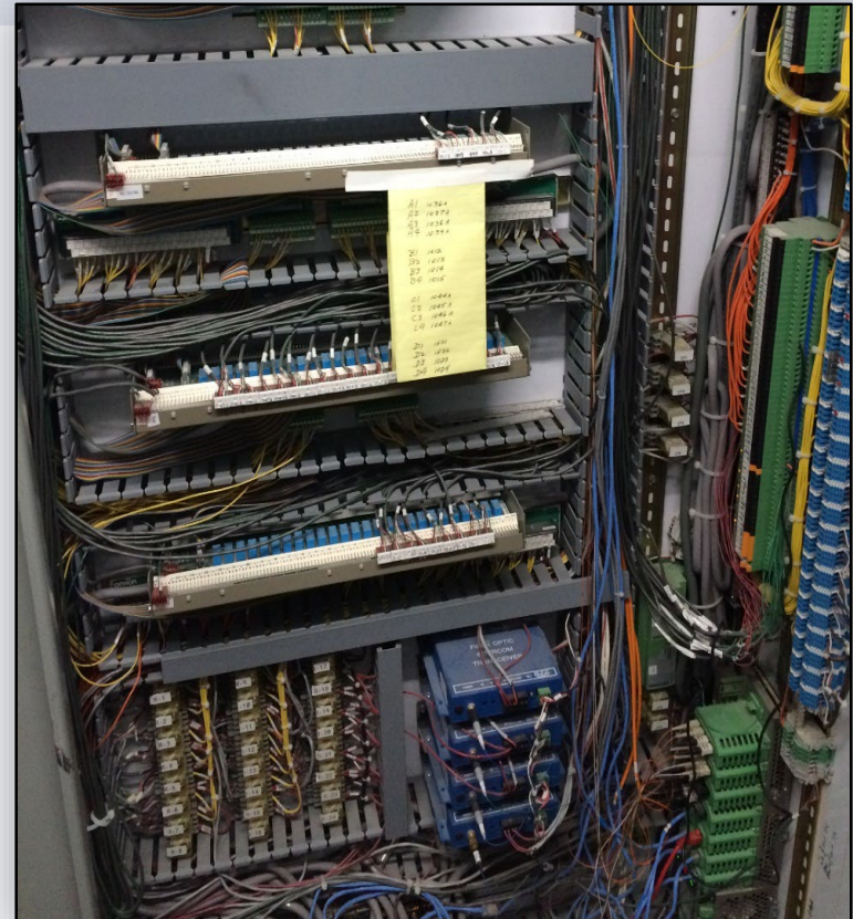
Arkansas Valley Correctional Facility Electrical door controls conditions
